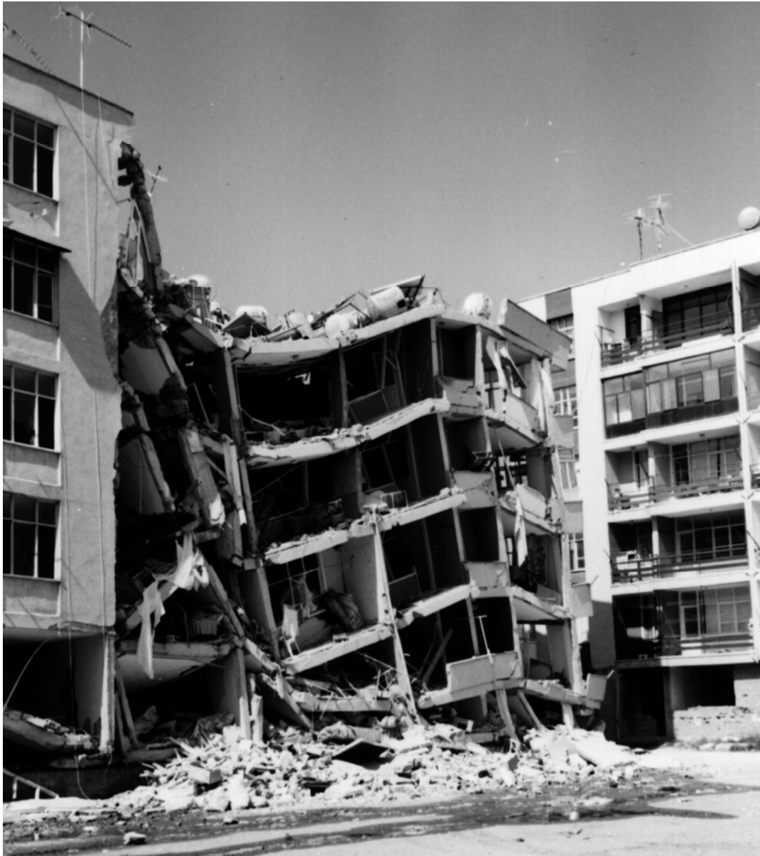
Figure 6: Partially collapsed building, due to the succession of flexible and rigid structural elements.
